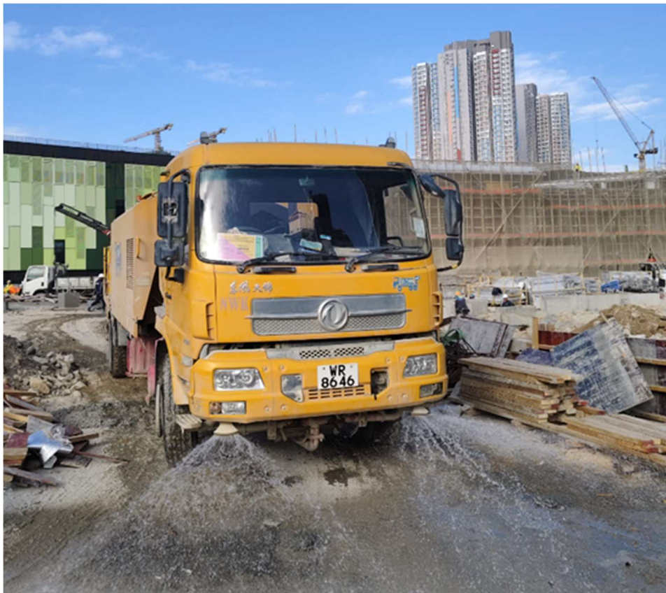
Photo 6: Water spraying truck has been provided on haul road to maintain wet surface.
